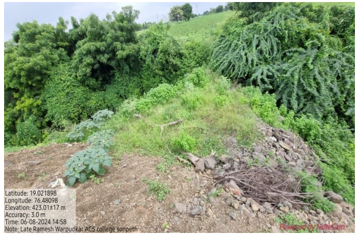
Rain water and waste water blocked
