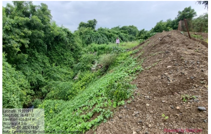
Rain water and waste water blocked
